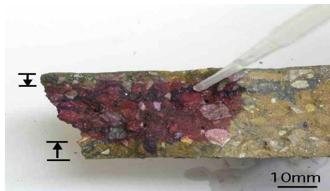
Fig. 6 Phenolphthalein indicator solution applied to a fresh fracture surface through a concrete slab.
